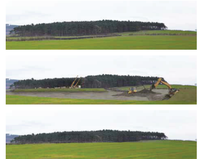
Illustration of construction impact at an MTS access point – before, during and after
